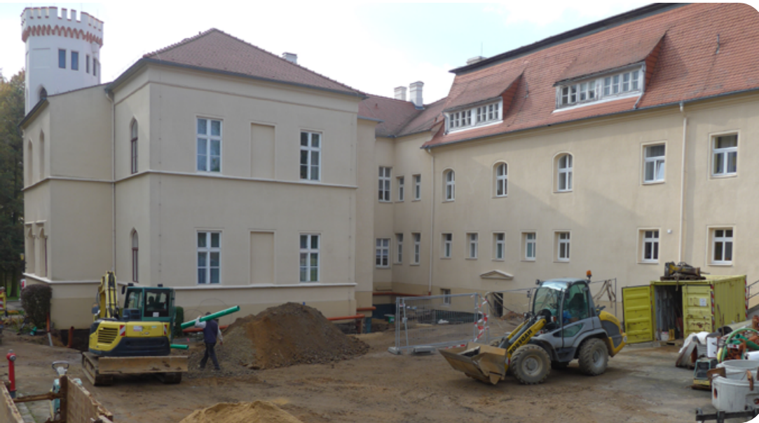
Preparatory constructions at the Caritas St. Hedwig North wing (Image credit: Caritas Association)
